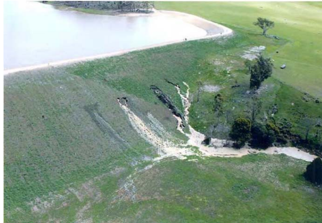
Barragens de terra – piping (ADSO, 2008)
